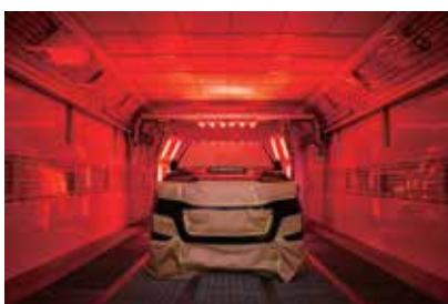
For measuring air velocity / Temp. in paint booth
